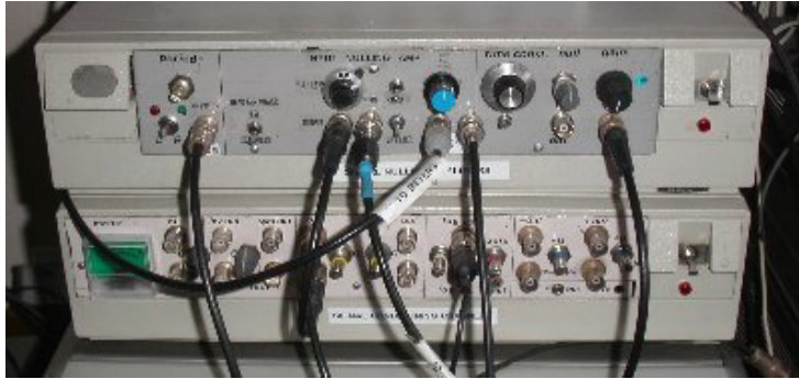
Figure 3 Post detector scaling and integration electronics
